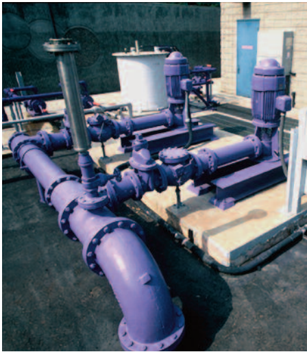
Recycled water treatment, storage and distribution are key components of NBWRP's Phase 1 projects.
