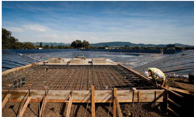
As part of the NBWRP, the Sonoma Valley County Sanitation District completed this reservoir storage project that provides storage of up to 100 acre-feet of water that can be used on a year-round basis by grape growers.
