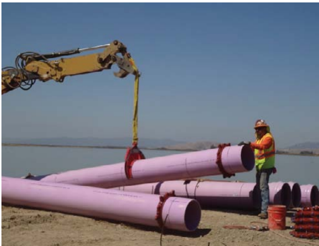
The NBWRP provided a 3.5-mile pipeline that carries water to a salt pond that is being restored as part of the Napa-Sonoma Marsh Restoration Project. The recycled water is also available to grape growers along the route in the Napa Cameros region, where water is scarce.
